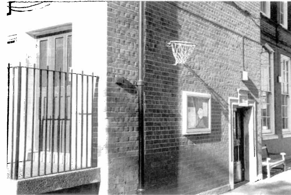
Figure 1.7 This Board School of 1910 has larger and smaller entrance doors for infants and juniors. (Photo: © Mark Dudek.)
