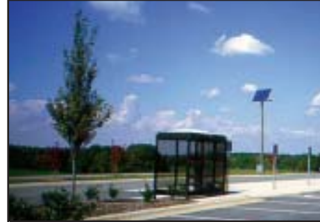
These stand-alone photovoltaic systems power parking lights.
