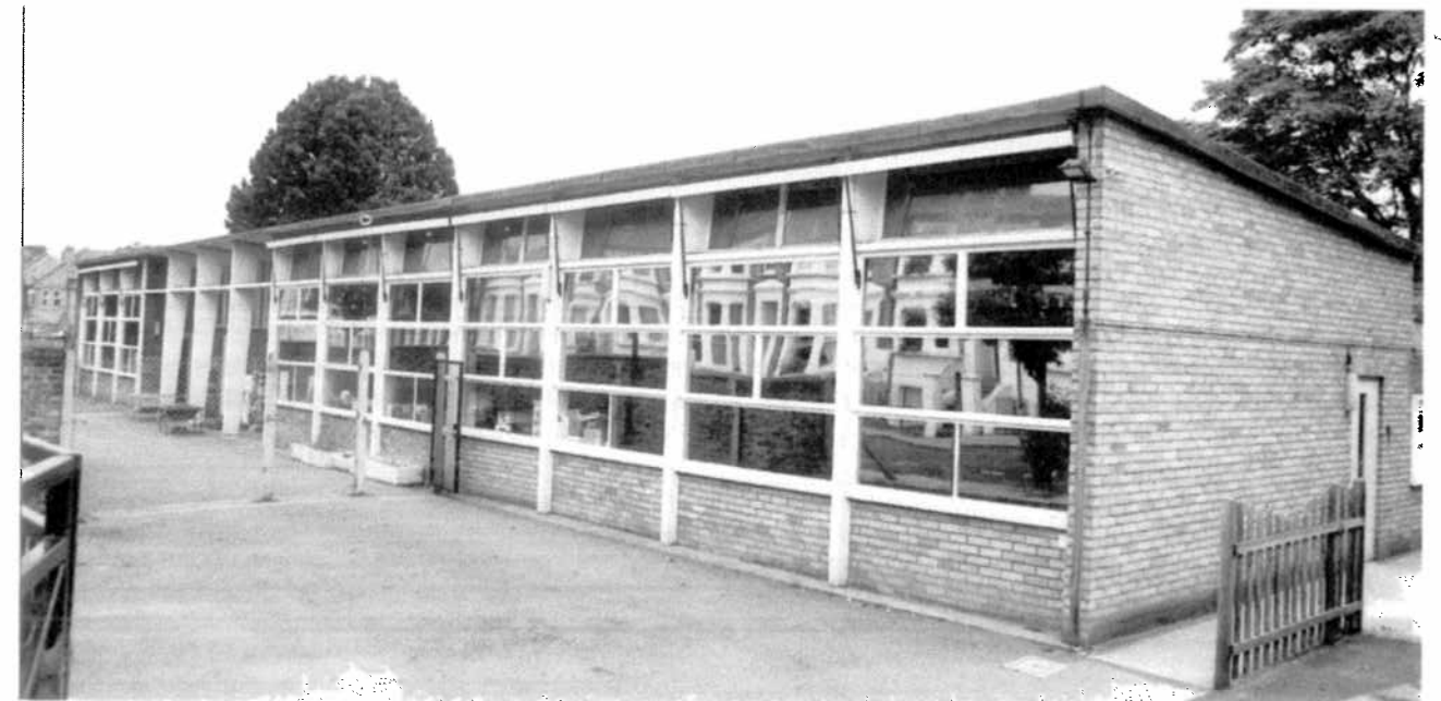
Figure 1.6b The school as it is today. With its draughty single-glazed windows and poorly insulated roof, the fabric does not meet modern environmental standards; its prefabricated form of construction makes it difficult to refurbish, however its organization and internal scale works well. (Photo: © Mark Dudek.)
